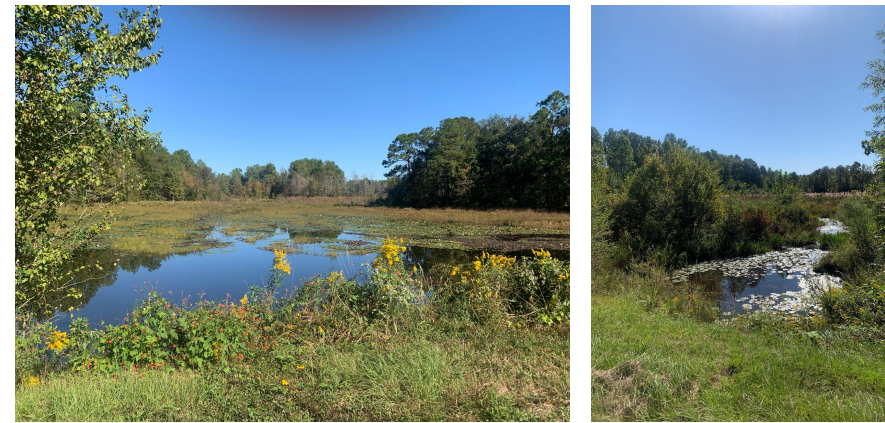
LEFT: Leftmost picture is the tributary upstream of the crossing at Lloyd Ave. in Reidsville, where water moves slowly through flat culvert, causing backups of water to pond as water moves down. Rightmost picture is the tributary downstream of crossing where it transitions back into a more defined channel condition.
