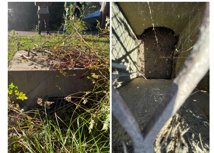
RIGHT: Debris within stormwater networks reduces capacity of infrastructure to collect and drain stormwater away from properties. Leftmost picture is of stormwater inlet in Collins, rightmost picture is of stormwater inlet along Chandler Ave. in Reidsville.
